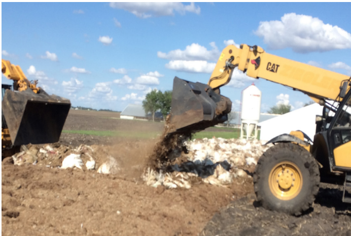
Figure 2. Combined materials being placed with a front-end loader and a telehandler from either side of the base without driving over it.
